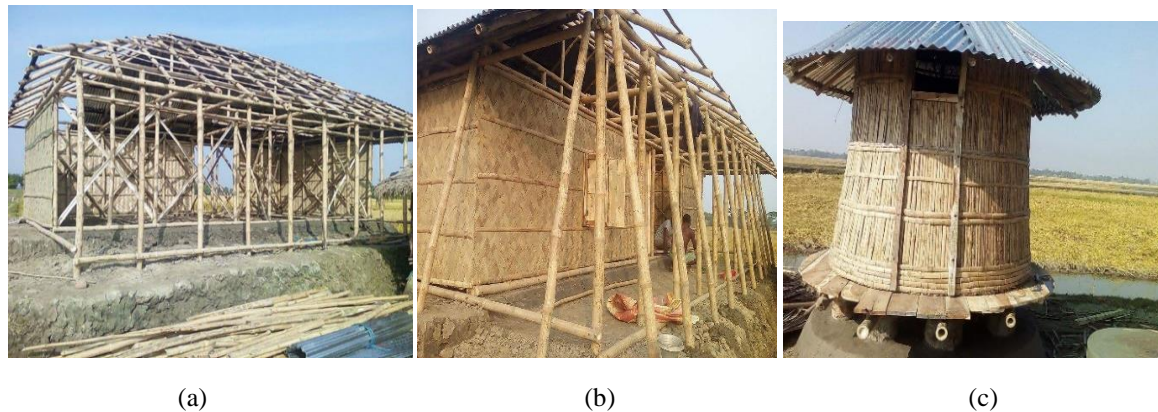
Figure 4. Implementation of design. (a) Structural frame of the house. (b) Structural buttresses to provide extra protection of the main structural system against strong and lateral forces. (c) Granary for food security.
